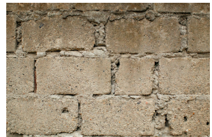
Brick Uneven Wall of Building in Street by Engin Akyurt, from Pexels
