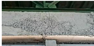
Concrete honeycomb on ring beam by Wikimedia Commons user, from Wikimedia Commons
